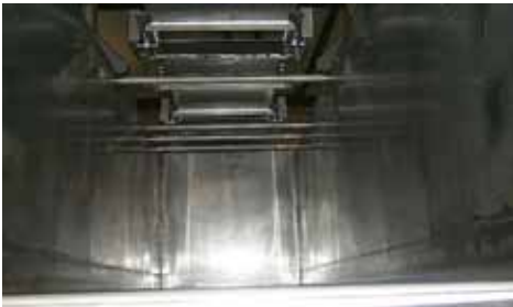
This accumulator is fit with a feed distributing conveyor mounted above the collecting trough.
